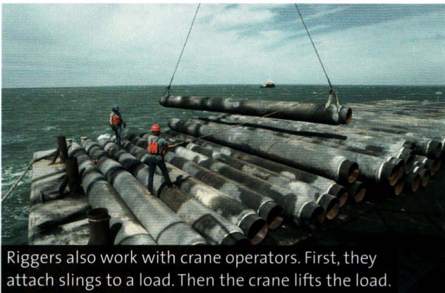
Riggers prepare lifting equipment. These riggers are erecting a rig to lift drilling pipes.
